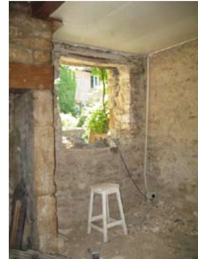
The plaster comes off then the window falls out and then the lintel turns to dust.
